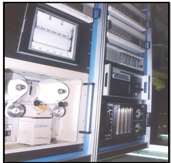
Figure 2: Continuous monitoring devices inside Misfalah station.
